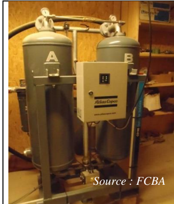
Air "drier" for compressed air compressor
