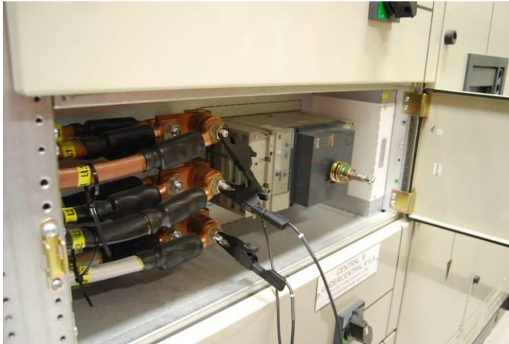
Figure 4. Mounting of voltage probes of a mobile meter in the electric central signal box.
